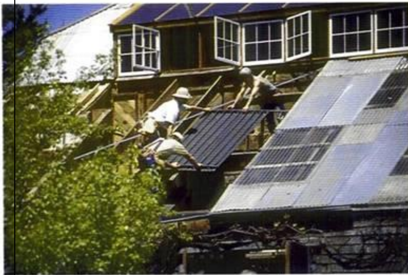
Workers install a roof-integrated solar hot water panel. Top Right: Sonoma State energy major graduates help install an integrated photovoltaics array.
